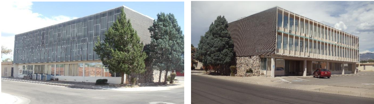
Figure 25. (left) Fox Building, North elevation. Note screens over the windows. (right) South elevation. Screens on this elevation have been removed.
